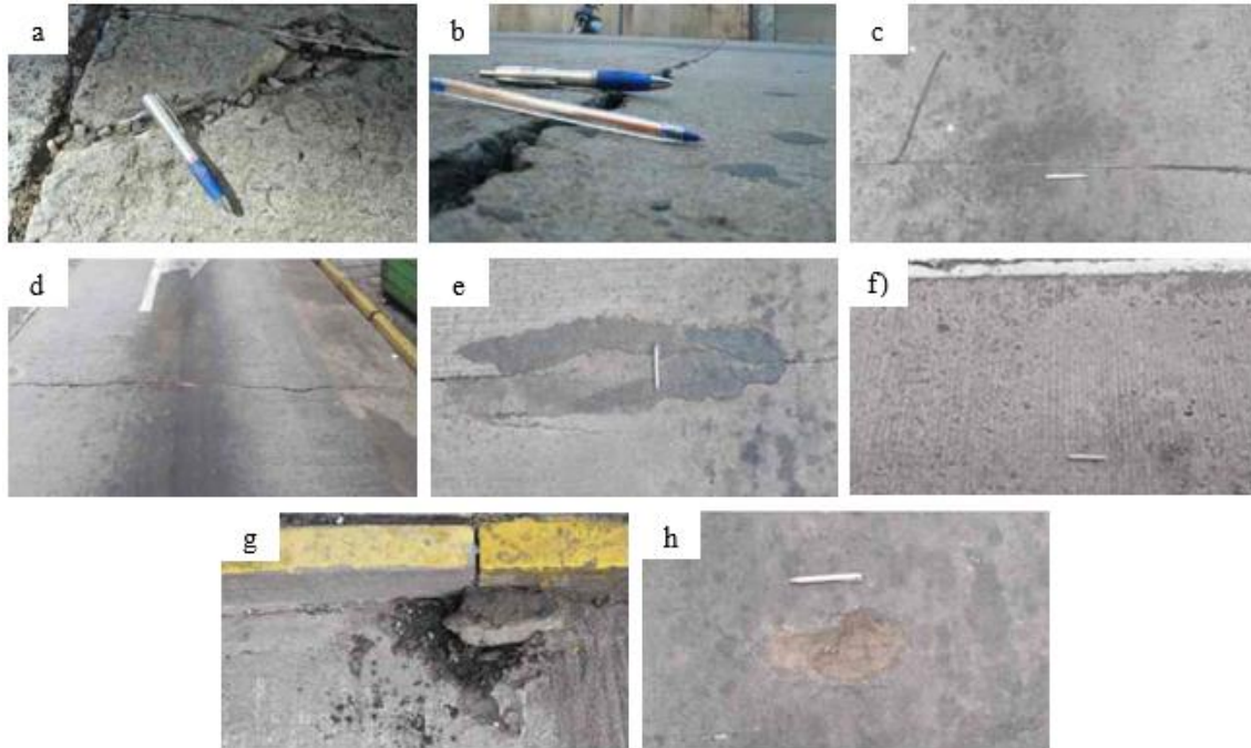
Figure 1. Main defects identified.
