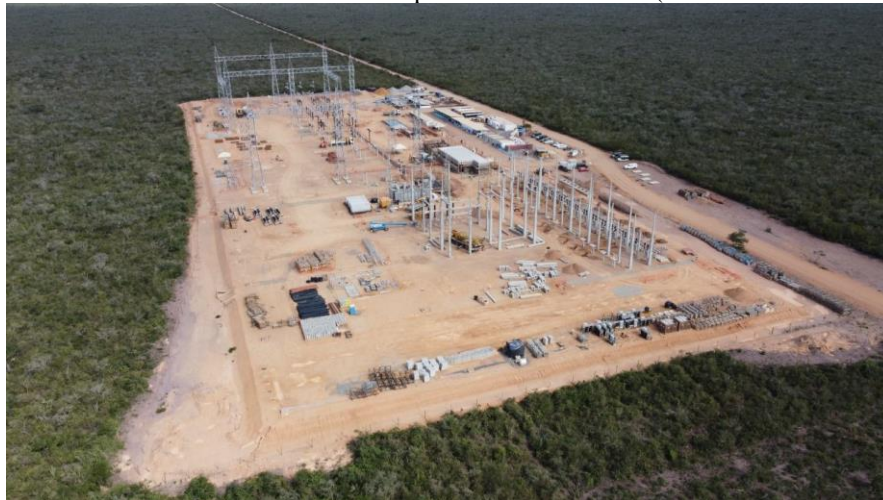
Figure 1: Construction site of the wind farm complex in Canudos- BA. (Source: From the authors, 2021)
